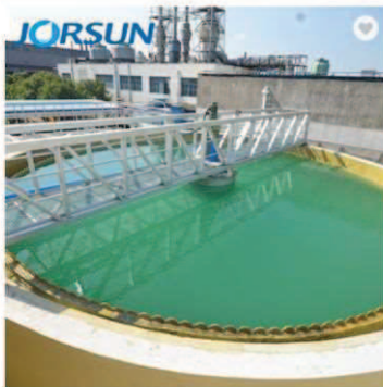
Full bridge sludge scraper used in secondary sedimentation tank
